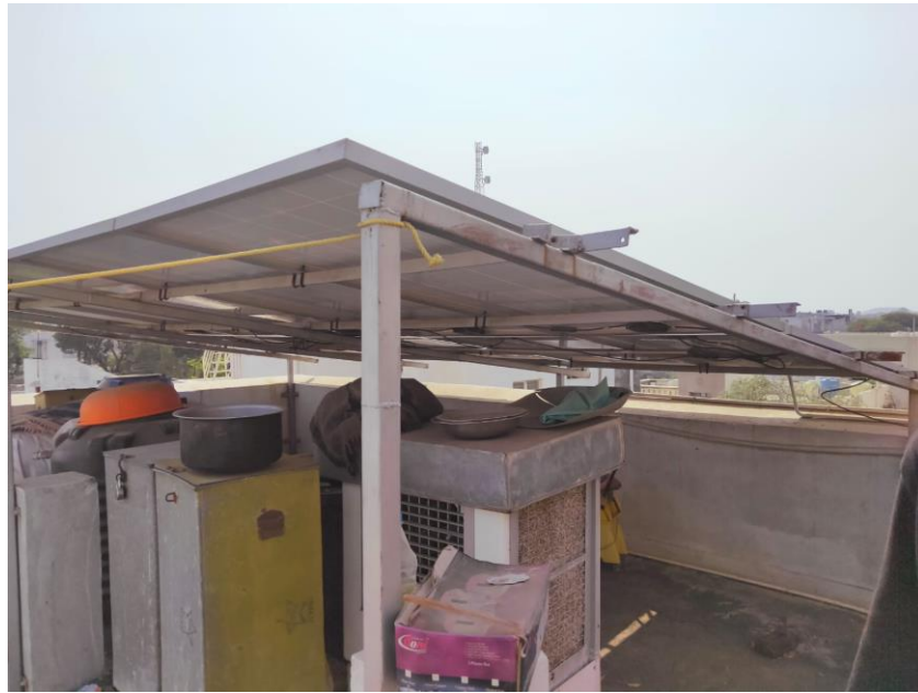
Fig.2 Solar panel placed at height
