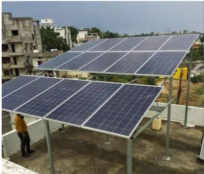
Fig.3 Solar panel at inclination
