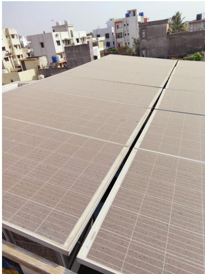
Fig.1 Solar panels in row
